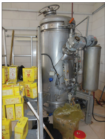
Figure 1: Hydroclave system in Shahid Rajaei Hospital and safety boxes
